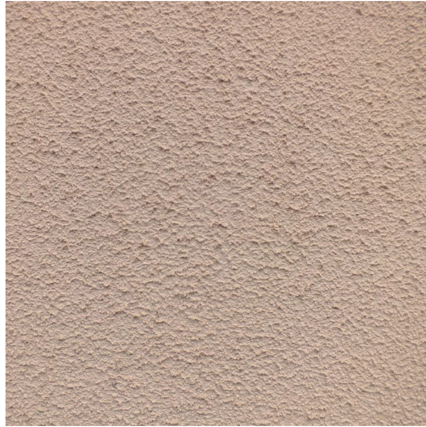
EIFS with stucco texture
